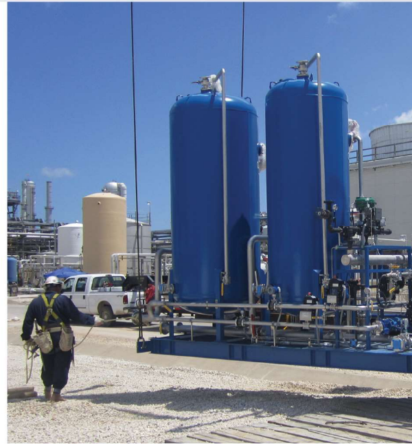
Culligan custom designed counter current, automatic demineralizer system built for Texas Chemical plant for process and boiler feed water.
